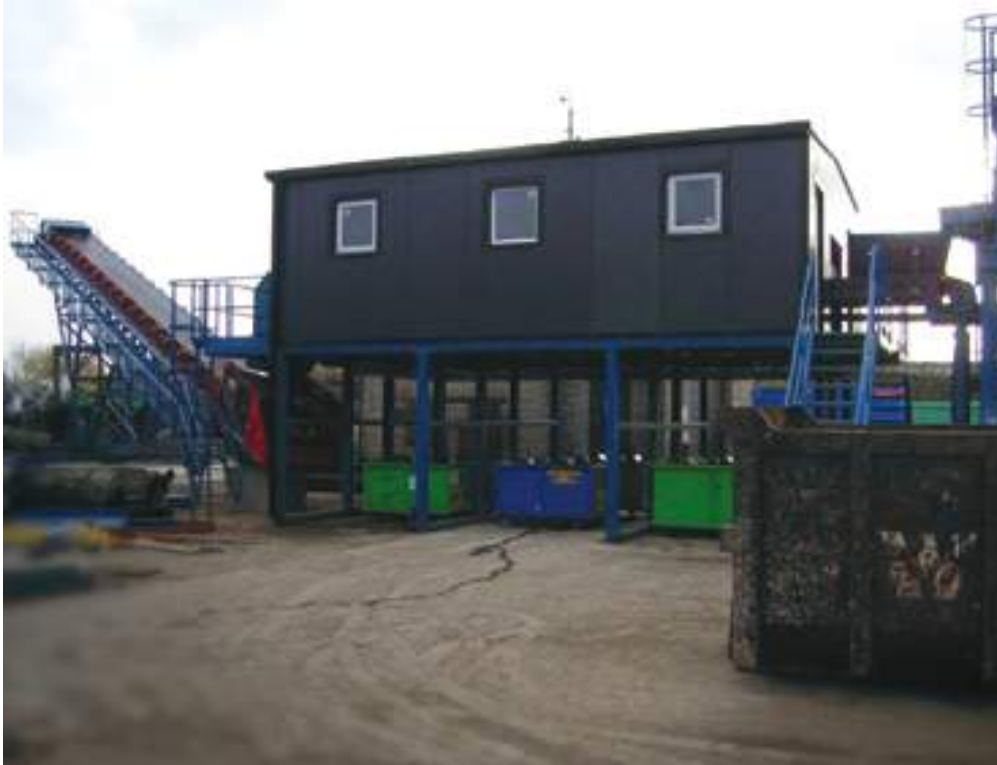
Picking Station and Radial Discharge Conveyor
